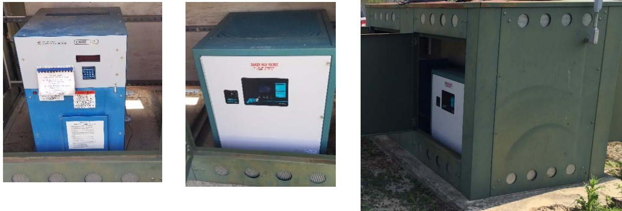
Figure 6: Existing Constant Current Regulators and Vault Enclosure
