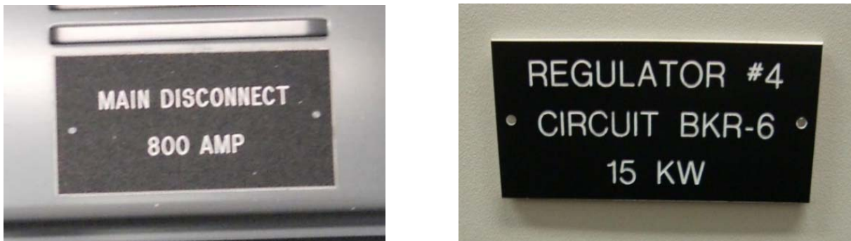
Figure 3: Typical Phenolic Nameplates on Main Disconnect and Regulator
