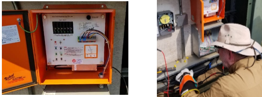
Figure 10: Pilot Control Lighting L-854 Radio Decoder
