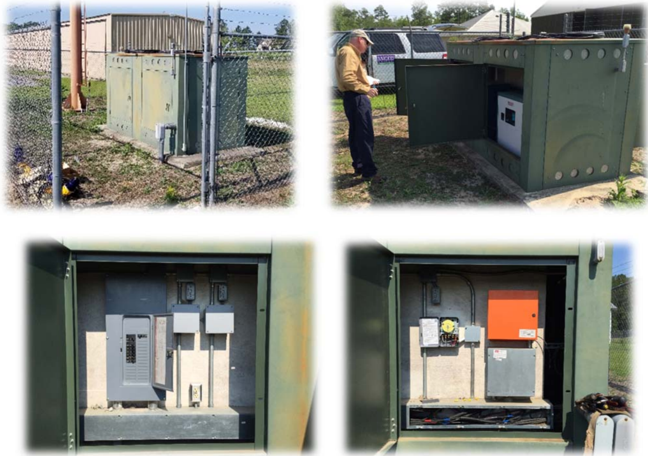
Figure 2: Airfield Lighting Enclosure (AFL Vault)
